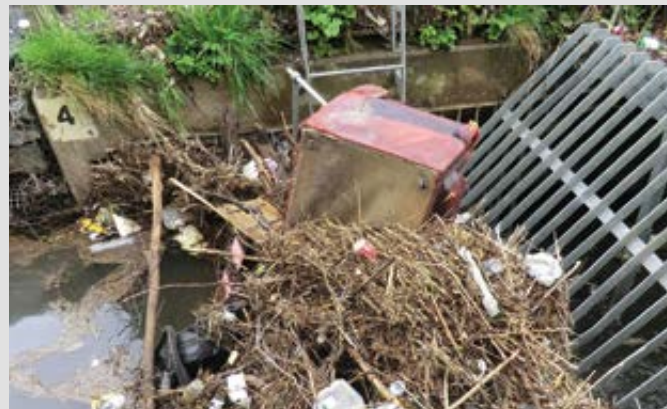
locked up culvert
